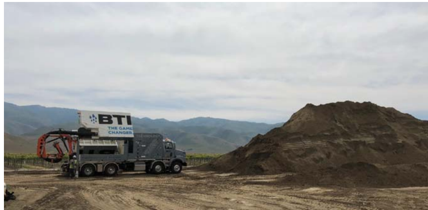
The Dino next to a stockpile of soil that it excavated. Excavated soil will be reused on-site.
